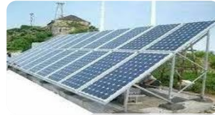
In-house Solar 2.4 MW (12%)
